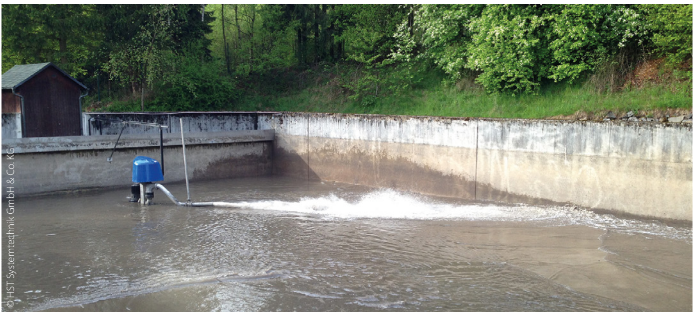
Figure 1: Swivel jet cleaner in a stormwater basin
